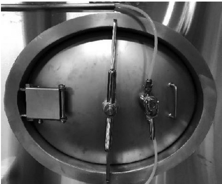
Sample extractor: mounted on manhole.
